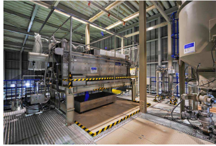
Fig.7 Inorganic materials separation pilot plant
